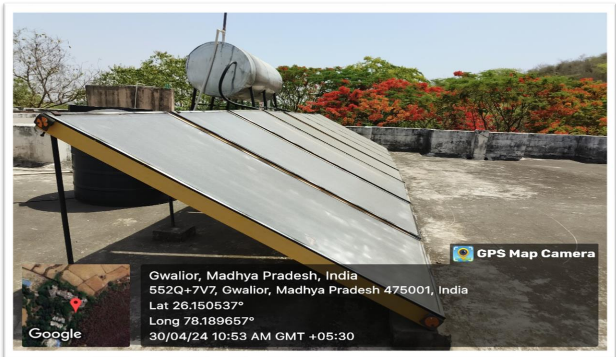
Solar water heating panels on hostel and residential complex
